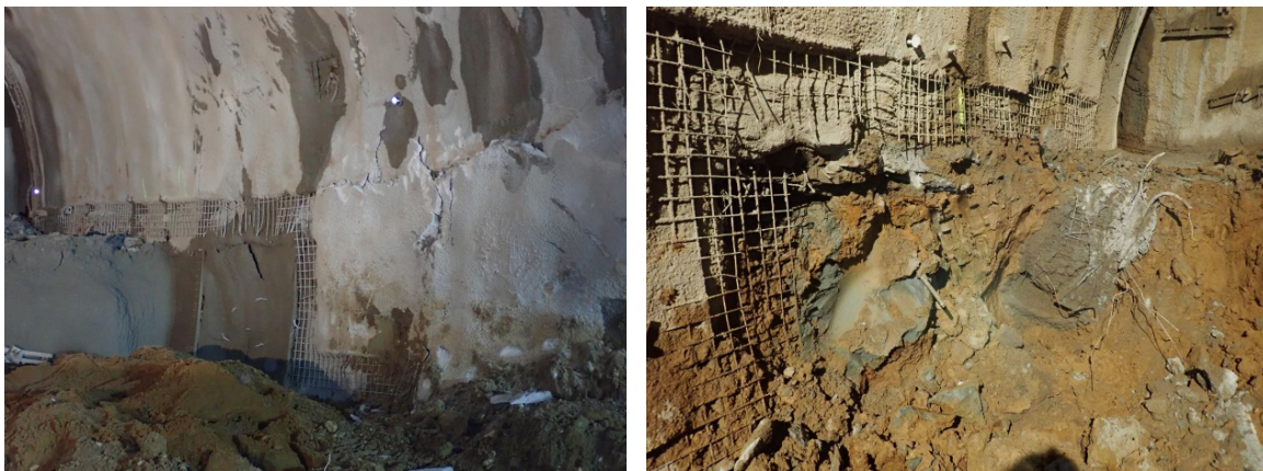
Figure 6. Crack formation/disintegrated shotcrete shell at chainage 85, right sidewall (left); left sidewall, bench excavation to chainage 94,3 – intact elephant foot and radial rock bolts of the top heading (right).
