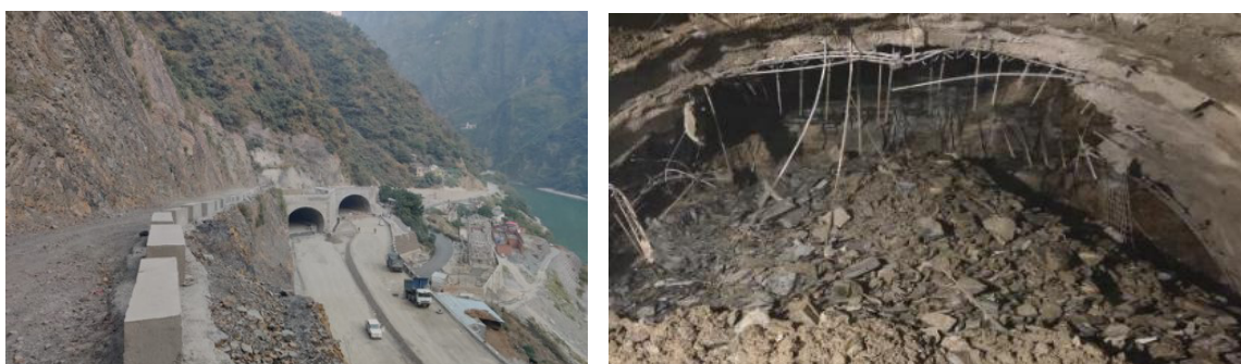
Figure 6. Tunnel T4-03 Western Portal (left) and overbreak in the top heading (right).
