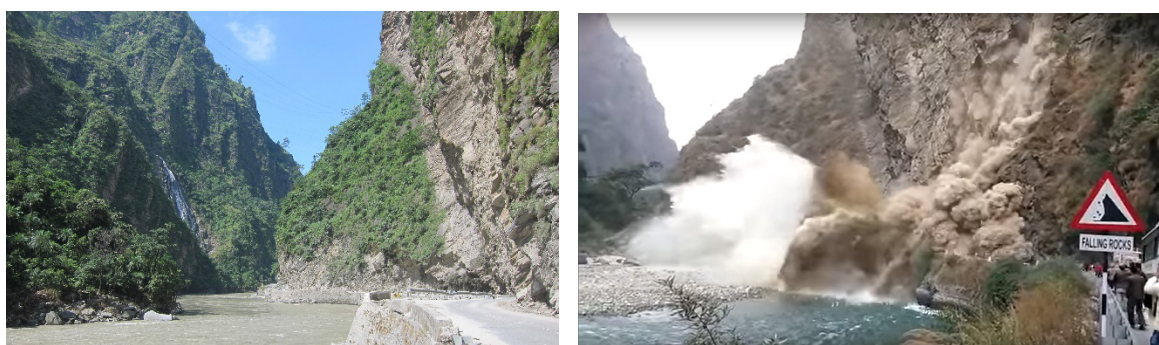
Figure 5. Steep natural canyon slopes parallel to tunnel T4-04 (left) with rock fall (right, from YouTube).
