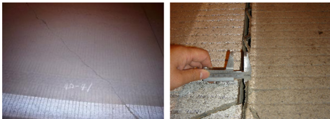
Figure 2. Damage of pavement concrete.
