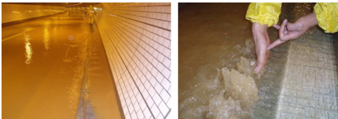
Figure 1. Flooding and groundwater inflow in tunnel.
