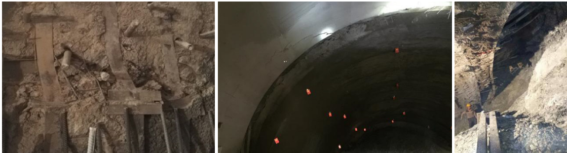
Figure 2. Severe extrusion and deformation of initial support.
