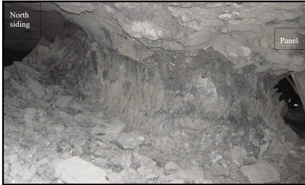
Figure 4. Pillar 13 showing more fracturing on the north siding side due to prolonged exposure.
