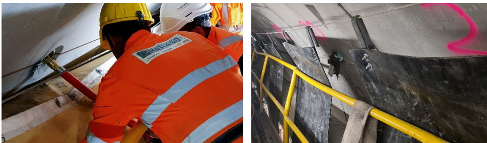
Figure 4. Left: Installation of receiver, Right: Shot holes with protective mats made from discarded conveyor belt material.
