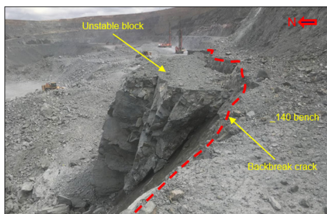
Figure 4. Example of slope instabilities (Sector 6).
