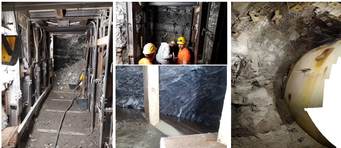
Figure 4. ET standstill at chainage km 17+332. Pictures of the lateral tunnel to free the TBM.
