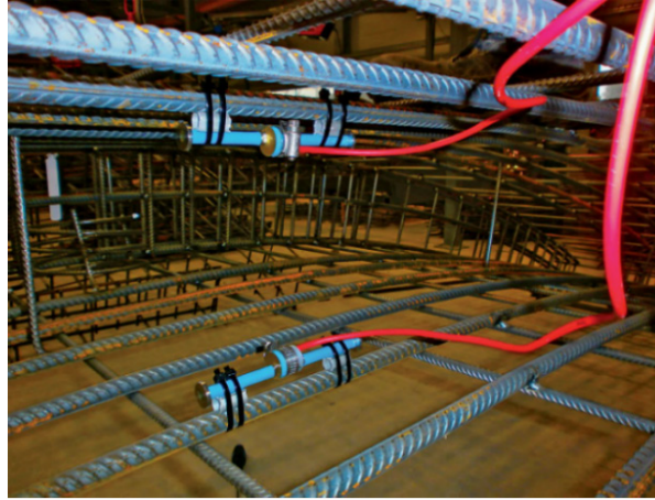
Figure 2. Vibrating wire strain sensors attached to circumferential reinforcement bars, before the placement of concrete (Radončić et al. 2015, copyright Ernst & Sohn GmbH. Reproduced with permission).
