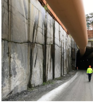
Figure 4. The boreholes of the experiment, Figure 2, partially intersected the rock volume where the entrance to the service tunnel was later excavated. The shallow, (sub)horizontal and large fractures are visible.
