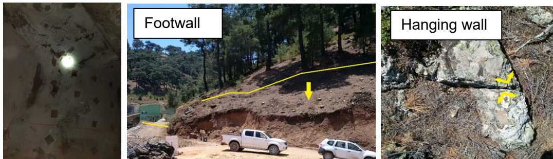
Figure 5. Underground cracks, the surface cracks on the footwall and hanging wall.
