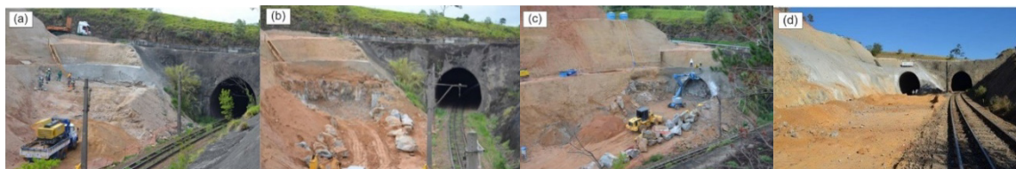
Figure 5. Photos of the portal execution steps in the specific tunnel – Source: authors.
