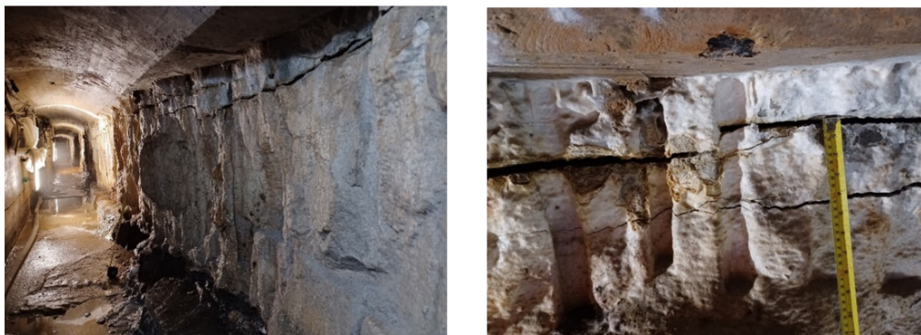
Figure 6. Subhorizontal open joints visible in the drainage tunnel at the concrete-rock contact.
