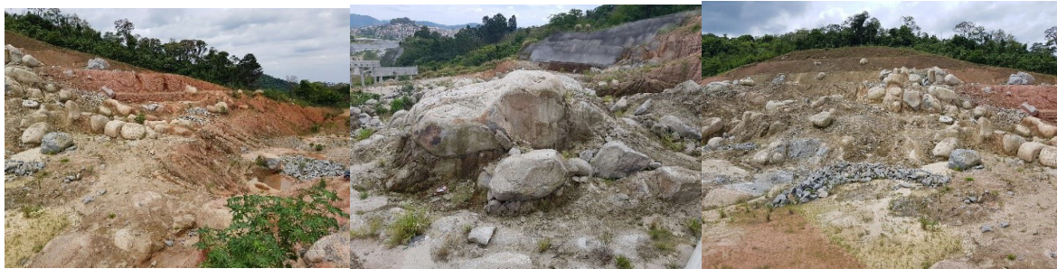
Figure 1. Places where the described methodology for boulders blast was applied – Source: authors.
