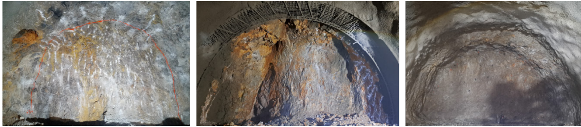
Figure 3. Photographs of tunnel face of the T1 main tube at chainages: a) km 4+473 local karstic feature in solid limestone; b) km 4+508 entrance to air filled cave; c) km 4+525 solid limestone.
