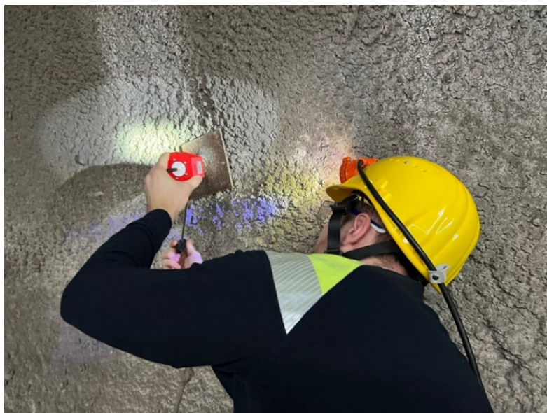
Figure 3. underground installation red type sensor bolt head, Breitenau mine, horizon X.
