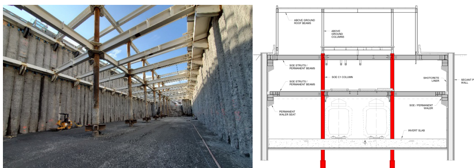
Figure 7. Permanent secant pile at Technoparc Station on the Airport Branch (Lee et al. 2022).
