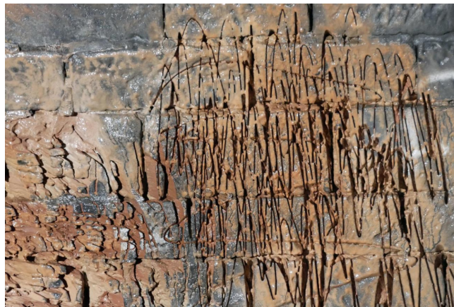
Figure 3. Surface of the masonry after tests with HPW cutting [source: Holzhäuser Ingenieur Consult GmbH].
