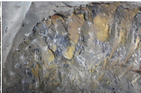
Figure 3. Face conditions in the top heading, comprising slightly to moderately granitic gneiss.
