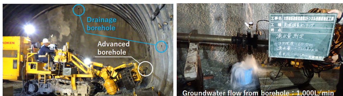
Figure 4. Photos showing the drilling operations and groundwater inflow near the tunnel face. (Left: Drilling drainage and advanced boreholes; Right: groundwater inflow from the borehole head)
