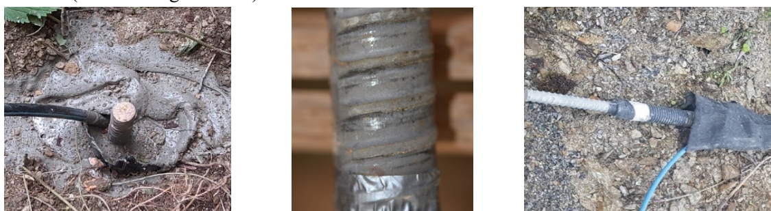
Figure 3. Examples for corrosion protection measures on micropiles, left: single corrosion protection using grout cover protection (GCP), center: single corrosion protection using zinc cover protection (ZCP), right: double corrosion protection (DCP).
