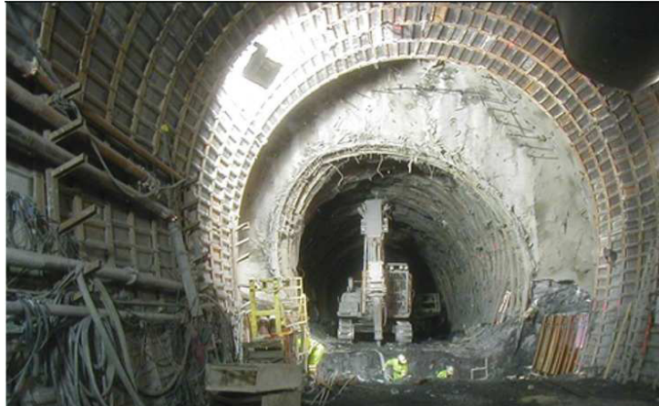
Figure 1. Squeezing closure of the Lyon-Turin Tunnel (Barla et al. 2008).
