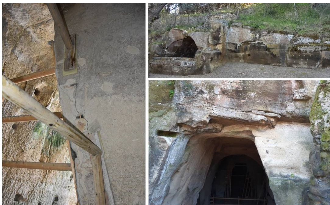
Figure 3. View of the cave and detail of natural joints and cracks caused by iron bar oxidation.
