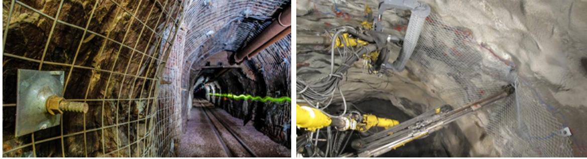
Figure 1. Ground support of a mining gallery with electro-welded steel mesh and high-resistance steel mesh in rolls, both fixed with bolts.
