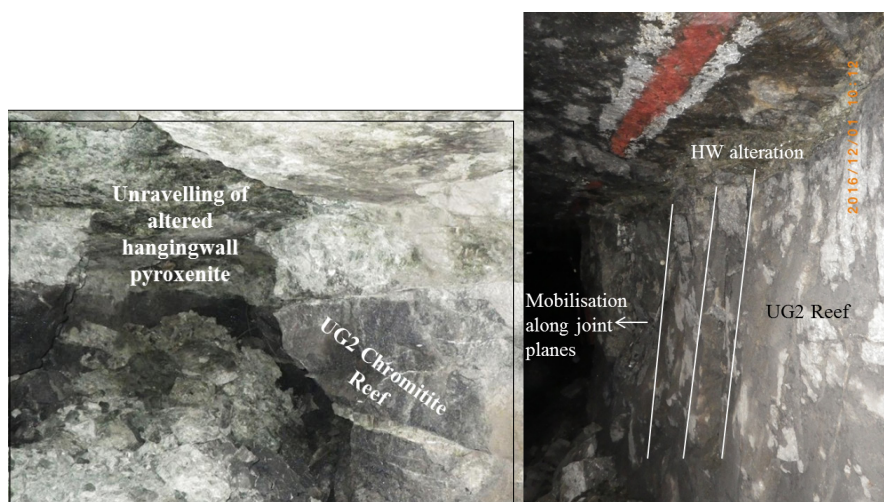
Figure 3. Left: Weak clay-like layer (alteration) zone exposed directly above the UG2 Reef, causing unravelling between installed support units. Right: Alteration along the top UG2 Reef contact causing mobilization along the joint planes. This led to pillar collapse.
