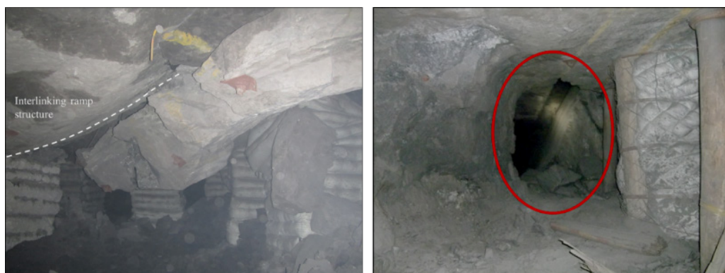
Figure 2. Left: Unstable hangingwall conditions in an underground stope panel where a low-angle ramp structure is present. The only support on the edge of this brow was in-stope rock bolt support and cementitious grout packs. Right: Panel instability shown at the red ellipse. Large-scale movement along a regional large-scale WNW-ESE trending fault structure caused a panel collapse.
